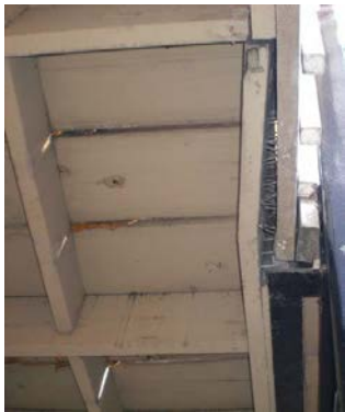
Walkway to 2nd floor becoming detached from support posts
