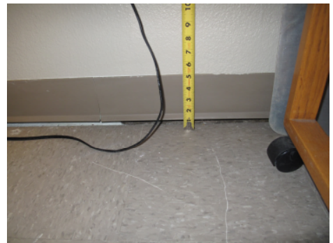
Vertical separation along the “trough”.
