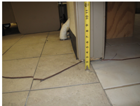
Vertical offset across cracked tiles.
