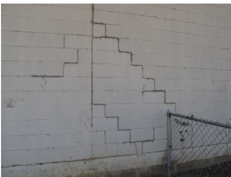
Step cracks in CMU wall at left side.
